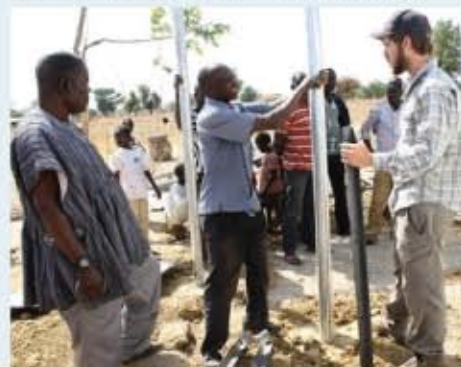
Matthew Petney works with local contractors on the support structure for the new water plaza. Photo by Anna VanMeter.
