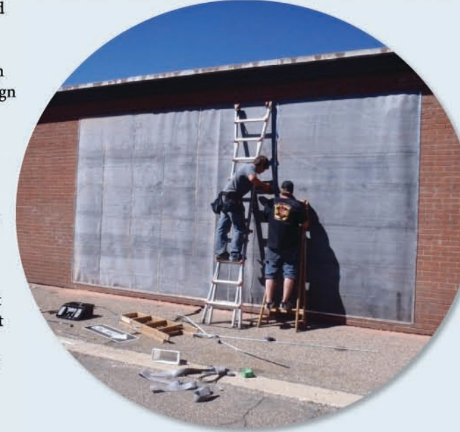
CM student Alek Herrick builds his solar heat exchanger at NAU Property Surplus.
